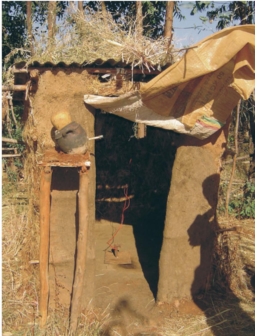
Figure 1 Demonstration latrine showing walls made from local materials, door made from recycled sacking material, a hand-washing station and a latrine cover.
