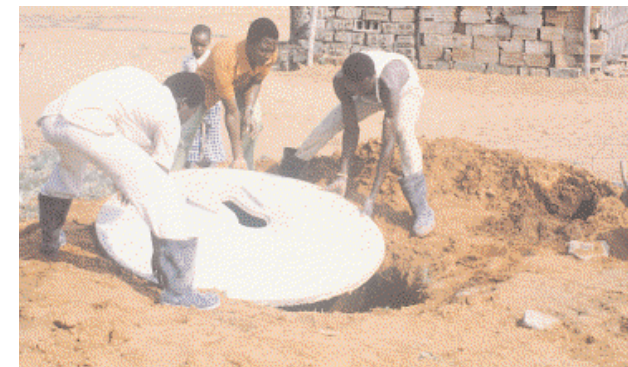
In Mozambique only, over 200 000 dome shaped SanPlats have been built using mainly the big 1.5 m type. In spite of its size a dome shaped slab is light weight and easily installed over a simple pit alone.
