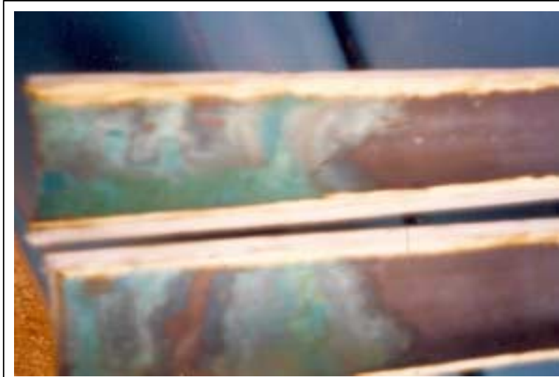
Figure 4. Corroded New Brass Cylinder Linings – Afridev
