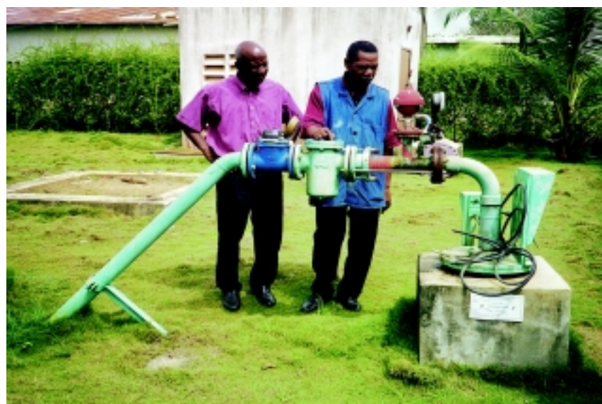
SODECI staff inspect the well-head at Songon Kassemble, Côte d'Ivoire.
