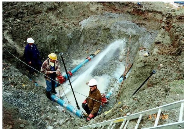
Figure 1 Simulated leak at test site as seen before ground reinstatement
