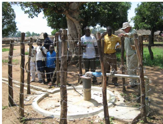
Plate 7 ~ Borehole Head at Patongo Camp
